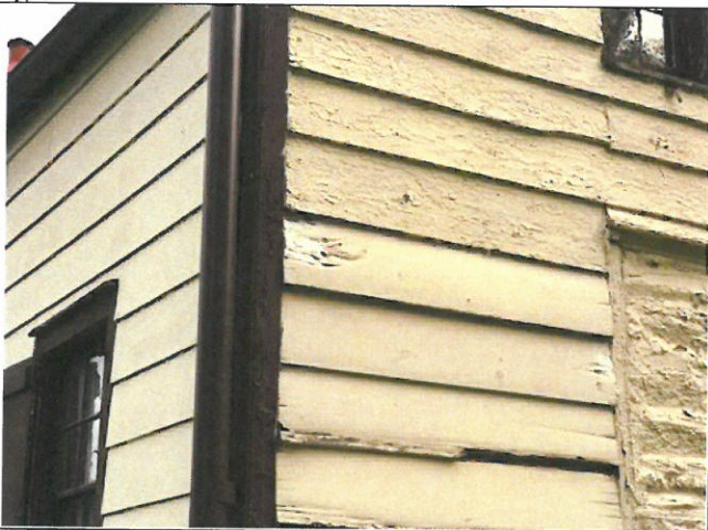
Photo 34. Area A, northwest corner, siding deterioration, typical.
