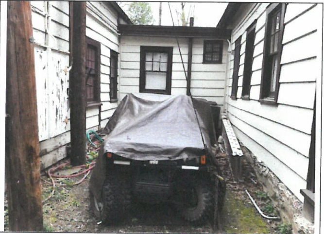
Photo 25. Area A on left, Area B connector ahead, Area C on right. Extensive drainage issues have caused foundation and sill damage.
