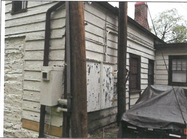
Photo 24. Area A, north elevation; Area B connector at right. Extreme drainage issues these sections of building.
