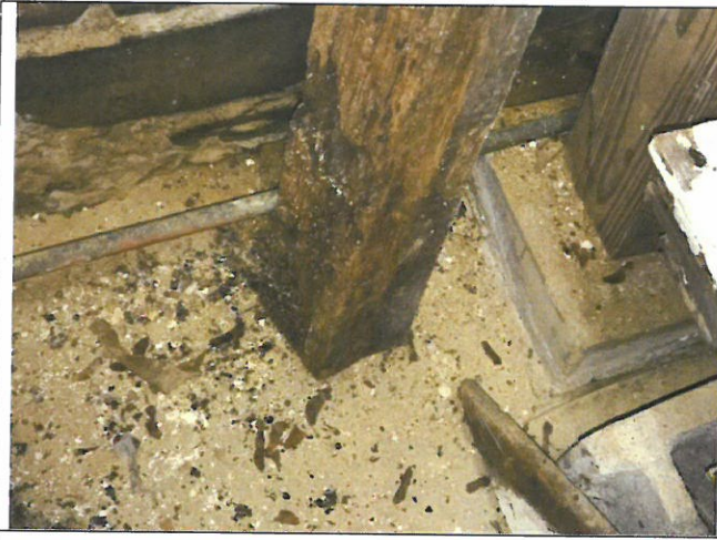
Photo 66. Area D, Room 001, southwest corner, evidence of infestation and deterioration, likely due to stored wood materials.
