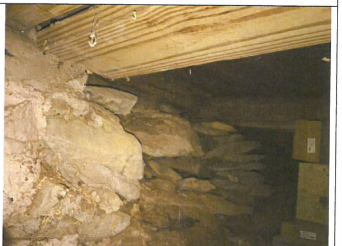
Photo 75. Area C, Room 105, view of replaced wood framing on stone wall in crawlspace, north wall.
