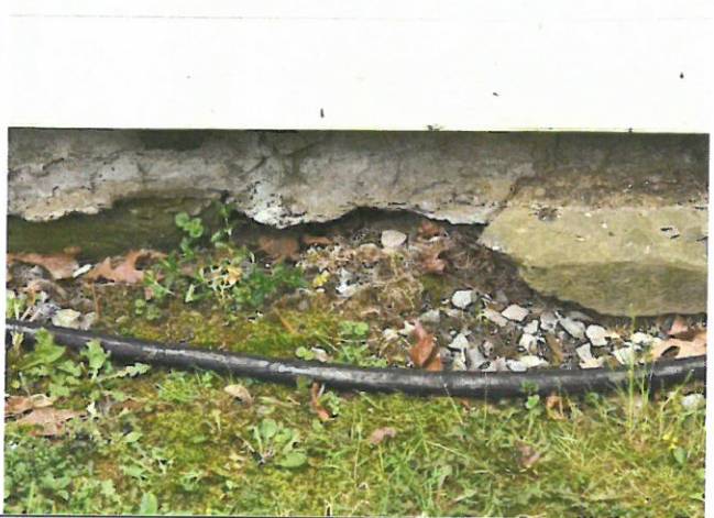
Photo 33. Area A, deteriorated foundation parging, typical.
