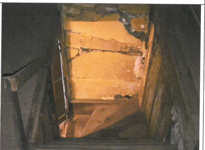
Photo 47. Area A, extreme deterioration (open to exterior) at south wall at base of stair, south elevation.
