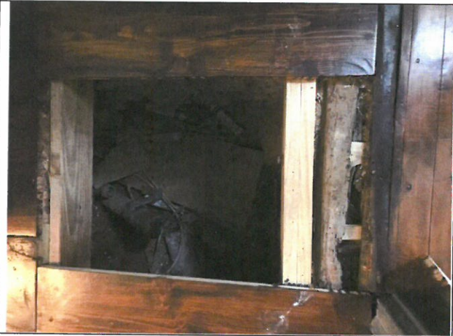
Photo 74. Area C, Room 105, opening in floor to crawlspace.
