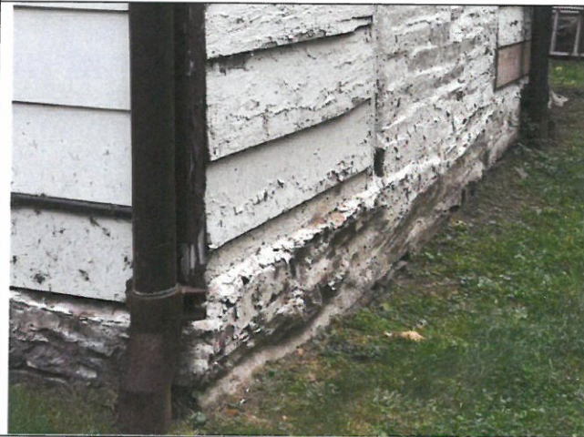
Photo 32. Area A, northwest corner stone foundation deterioration, typical.
