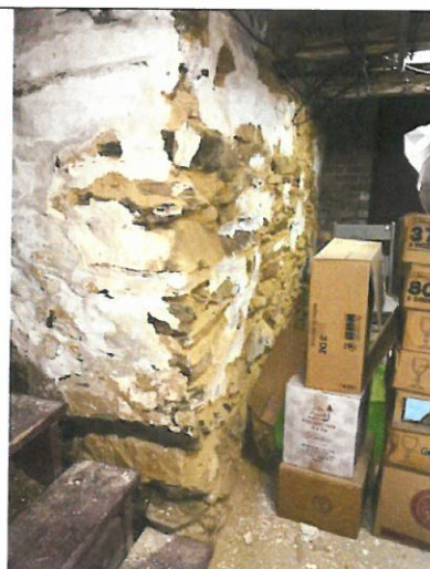
Photo 65. Area D, Room 002, loose and spalling stone at Stair 2.
