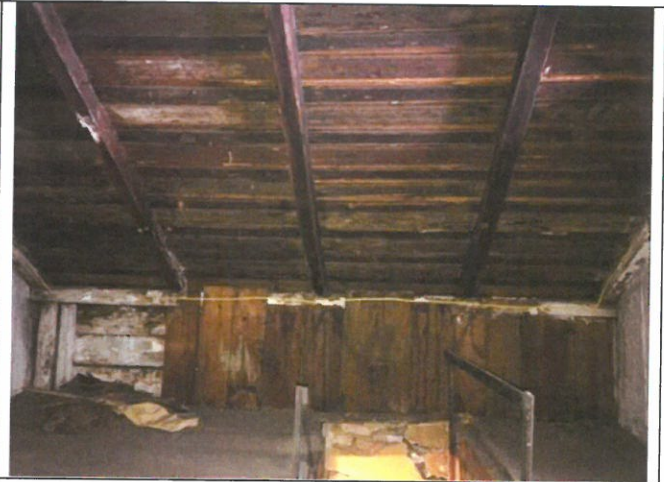
Photo 55. Area A, Room 202, condition of roof and wall framing, typical.
